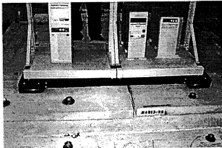
Figure 7 - LAN rack with base isolation
